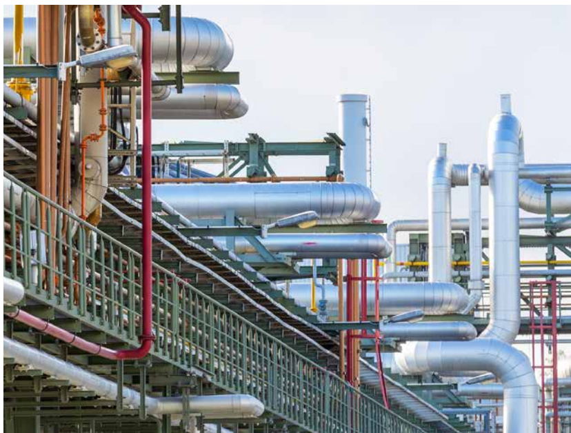
Thick sets of pipes transport raw materials, byproducts, products, steam and production-plant media exactly to where they are needed. The integrated production approach of German chemical sites has been very successful since the 1990s.
