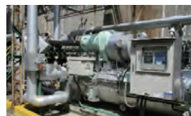
Fluorocarbon cooling equipment
