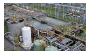
Activated sludge treatment facility
