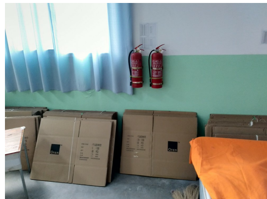
Blocked fire extinguishers 2 fire extinguishers in the packaging area were blocked.
