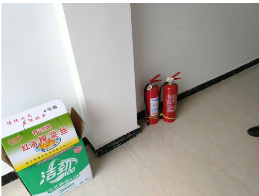
Fire extinguisher placement 2 fire extinguishers in the kitchen were placed on the ground.
