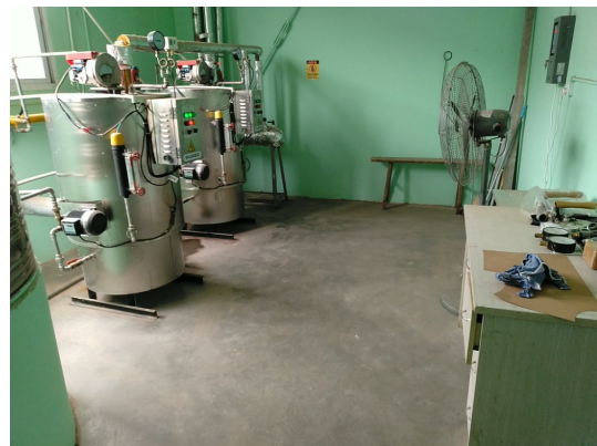
No fire extinguisher No fire extinguisher was available in the boiler room.
