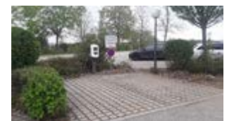
Charging station (Germany)
