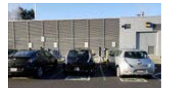
Charging station (United States)
